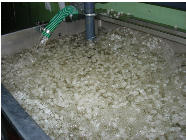
Moving Bed Biofilter
